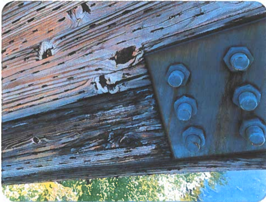
Photo 4: Northwest arch splice cracking
