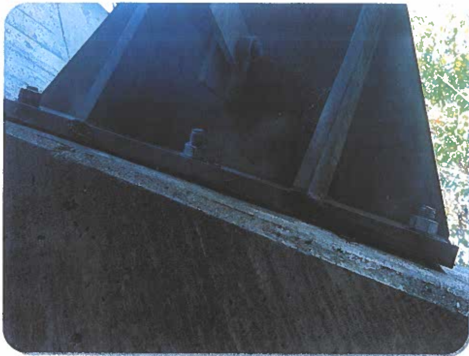
Photo 19: Debris underneath bearing.
