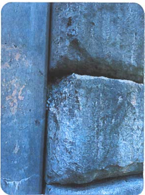
Photo 24: Modular block deterioration.
