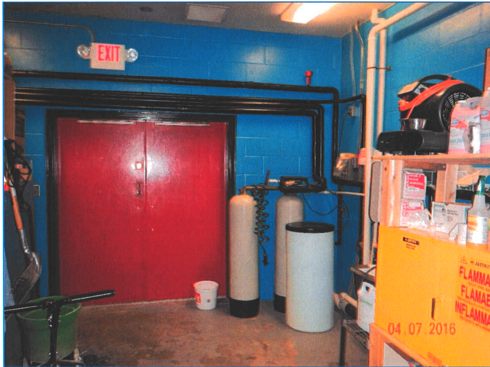
Mechanicals Room REQ
