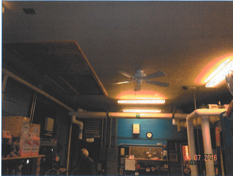
Mechanicals Room REQ
